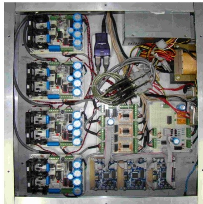
Figure 2. Power and electronic control module (PECU) cabinet, completely designed for the automation of the Cartesian robot.
